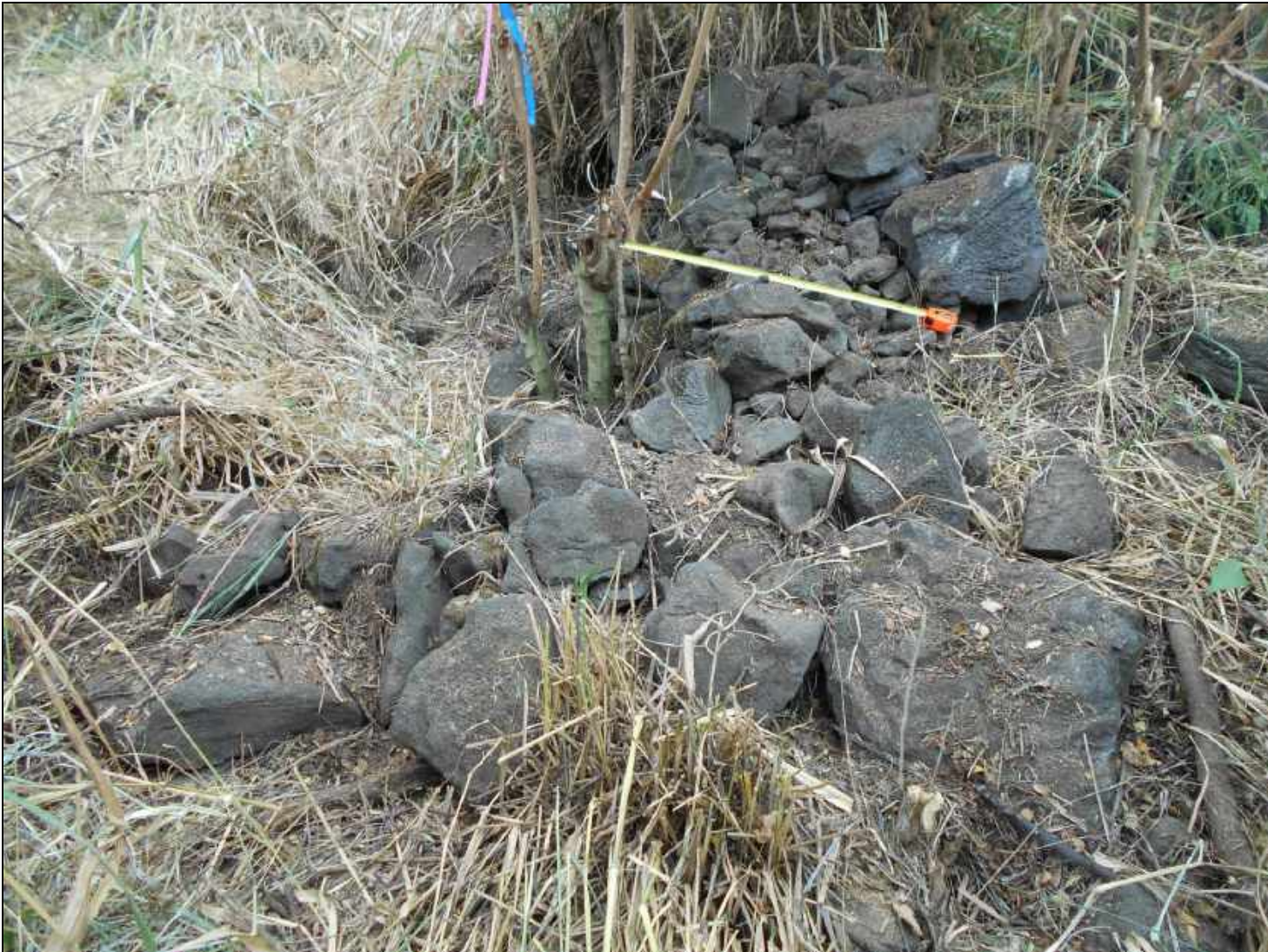
Figure 27: Photograph of Site 30595 Wall Collapse Showing Cobble Core Fill, Looking North.
