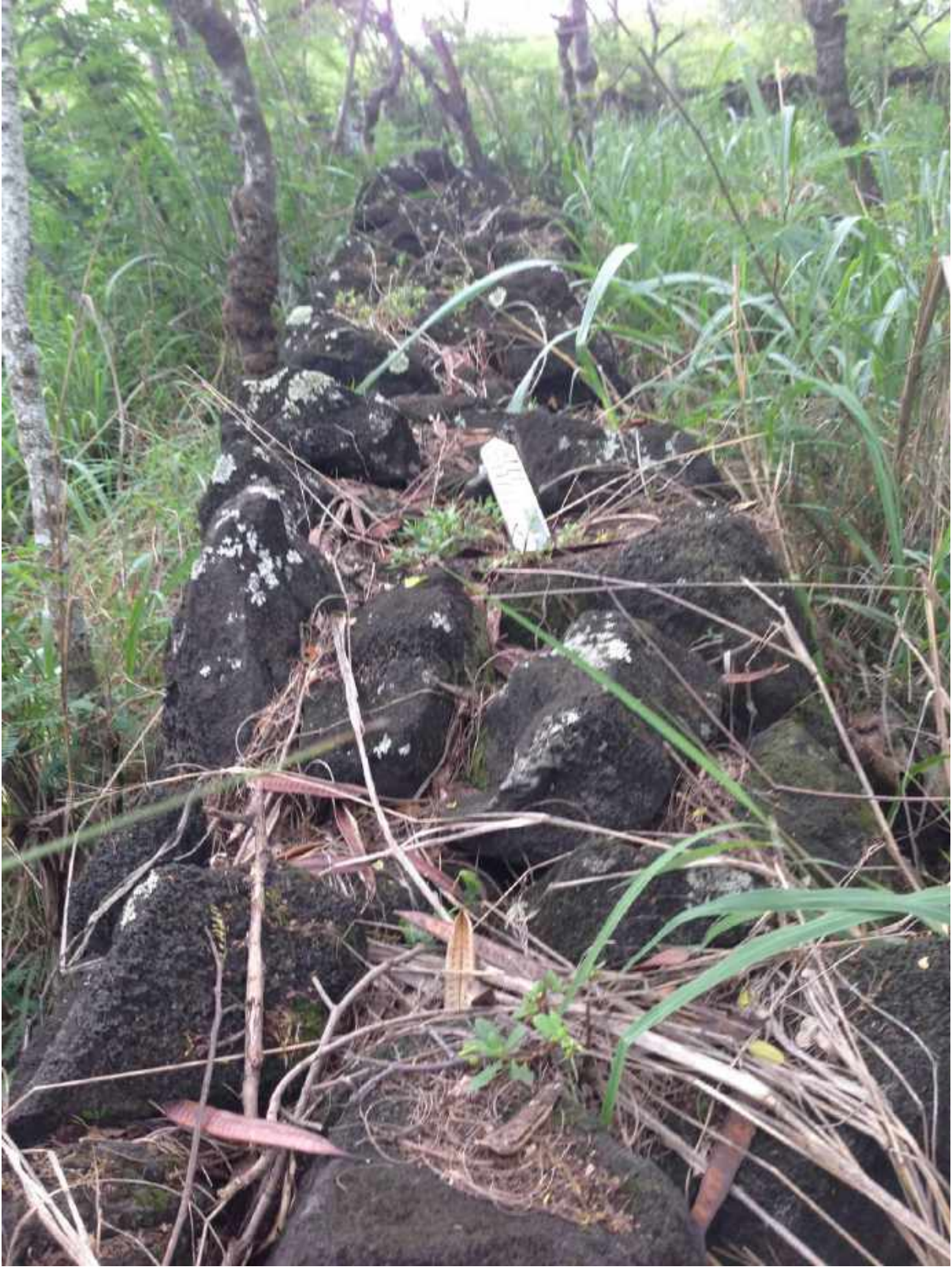
Figure 72: Photograph of Site 31182 Feature 11 North End Showing Top of Wall Construction, Looking North.
